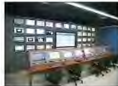
Monitoring and Service Center for Internet of Things in Agriculture
